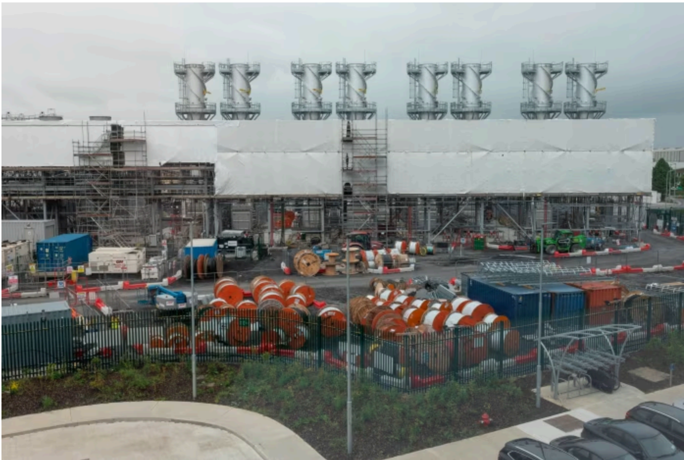
Gas turbine exhaust stacks on the campus being developed by Echelon, one of Europe's largest data centre operators © Paulo Nunes dos Santos/FT
